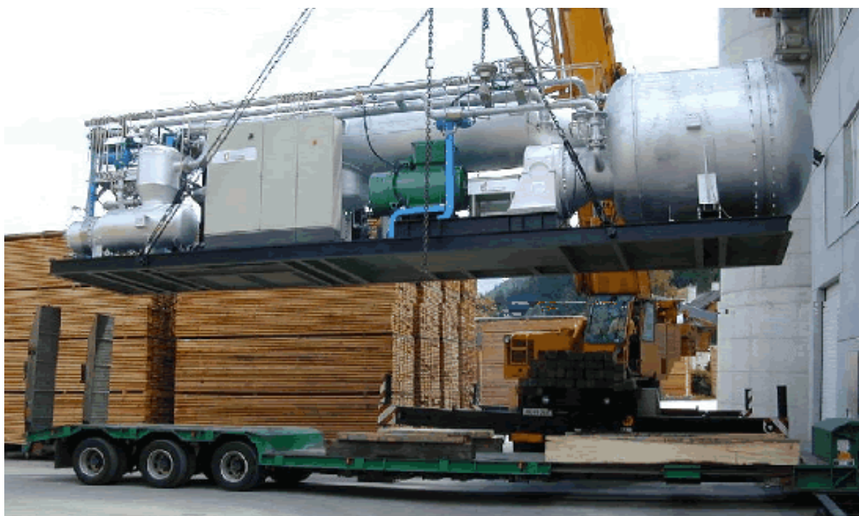
Figure 15 : An ORC power plant 20 ; Source :Turboden, Brescia, Italy.
